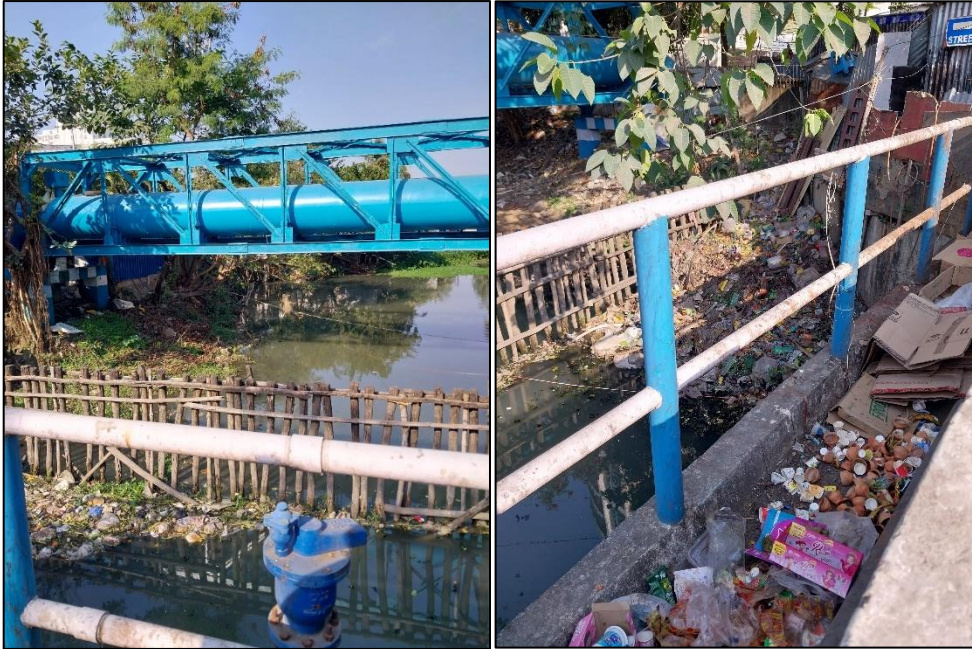
Figure 35: Clogged drainage system, causing inefficiency and reduced capacity during the rainy season. Source: Author, (2024)
