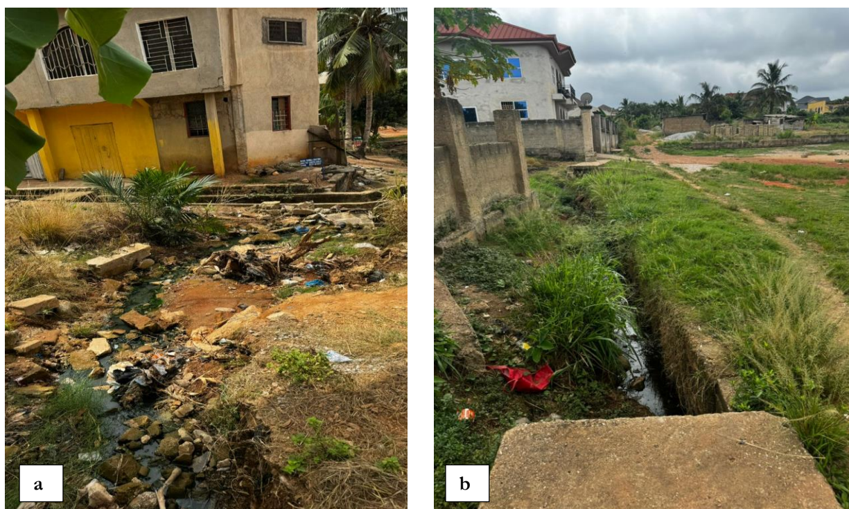
Figure 8: Small scale street drain unconstructed (image a) and covered with weeds (image b)
