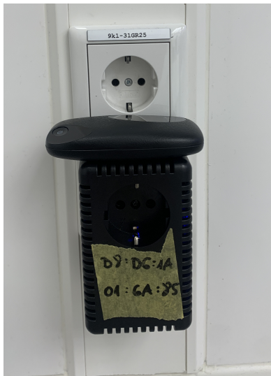
Fig. 13. Power Quality Monitor #2 and TP-Link Mifi Router
