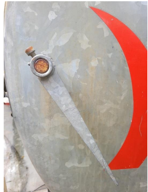
Figure 18, mechanical float mechanism indicating the water level inside the tank
