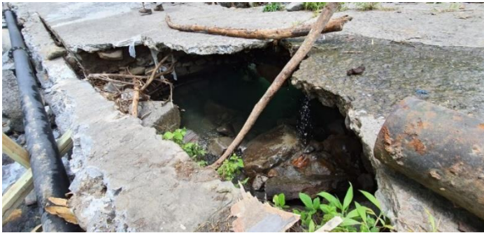
Figure 7. Damage to river crossing. (Courtesy: Antonia Marks, 2021)
