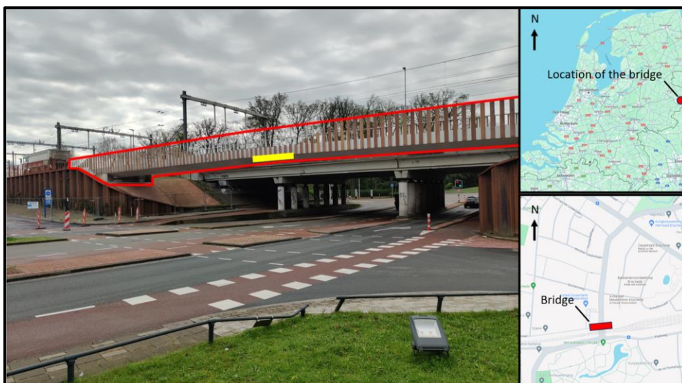
Figure 5: The F35 bicycle bridge across the Tubantiasingel: a photo of the bridge from north-west with the location of the TMD shown as a yellow box (left) and its geographical location (right)
