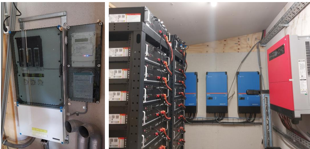
Figure 5: Aardehuis' new electrical panel (left), batteries and management systems (right). Taken by researcher.
