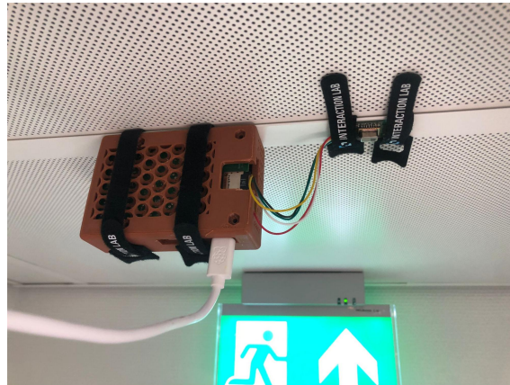
Figure 11: the sensor installation
