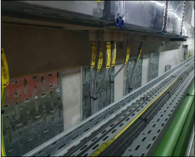
Figure 12: Coding on Cables of EHT
