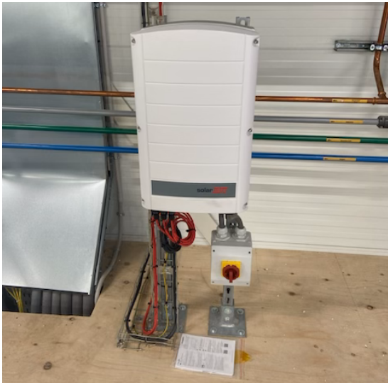
FIGURE 4.3: Inverter of the PV system of Fraunhofer Innovation Platform for Advanced Manufacturing.
