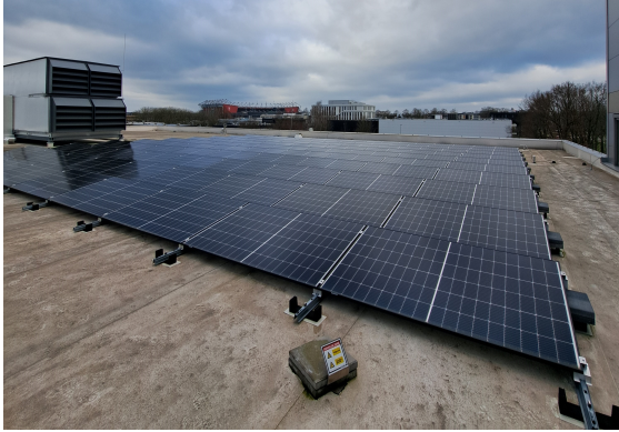
FIGURE 4.1: PV system on the rooftop of Fraunhofer Innovation Platform for Advanced Manufacturing.
