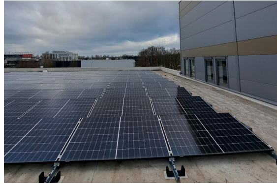
FIGURE 4.2: PV system on the rooftop of Fraunhofer Innovation Platform for Advanced Manufacturing.
