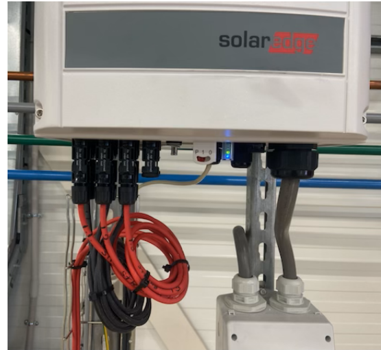
FIGURE 4.4: Inverter of the PV system of Fraunhofer Innovation Platform for Advanced Manufacturing.
