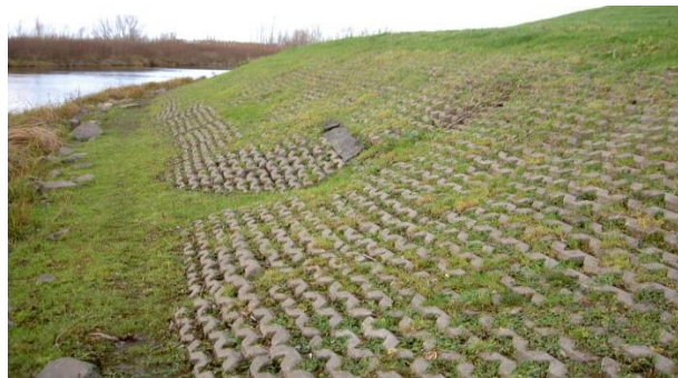
Figure 10: Grass paving revetment to prevent animal burrows at the Erlecomsedam (Waterschap Rivierenland, 2016).
