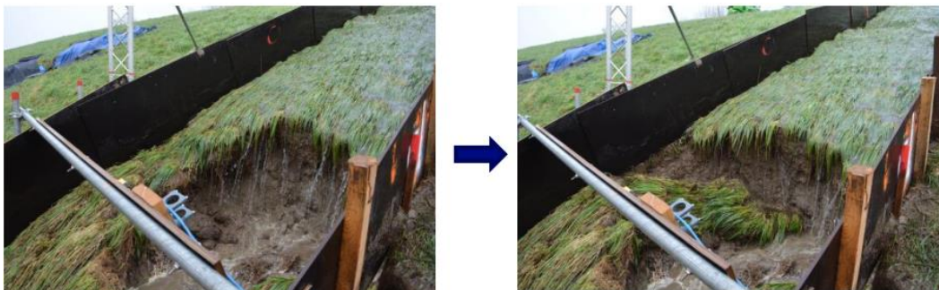
Figure 6: Erosion of the revetment layer (and the slope beneath) in an advanced stage (Deltares, 2023a).
