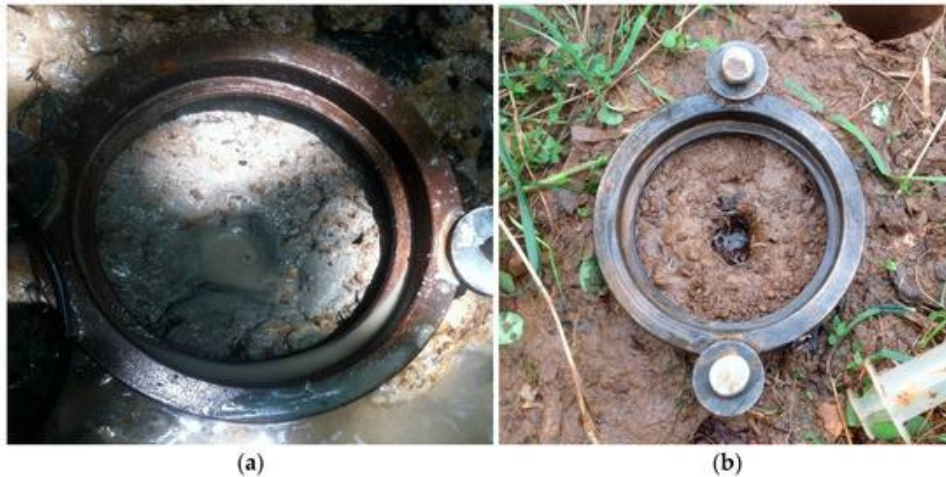
Figure 3 - Photos of scour hole formation in different soil physical conditions (a) wide and shallower, and (b) narrow and deeper (Mahalder et al. 2018).
