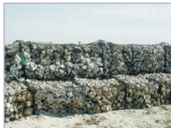
Figuur 18: Gabions noodmaatregel [Moore et al., 2014].
