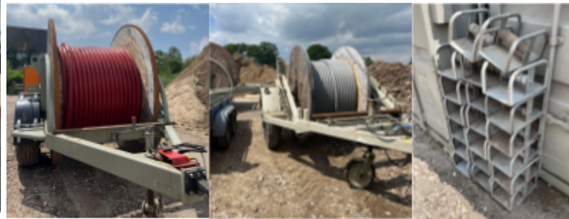
Cable is attached to a wagon. These are moved with a smaller truck into the site. Cables are later pulled with steel artifacts that allow an easier pull (Image 3).
