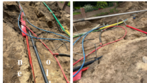
During the site visit it was possible to see how the new cable was being laid next to the old cable. It was also interesting the procedure on how the the new cable is laid, protected with the plastic red rug and then covered back with soil.
