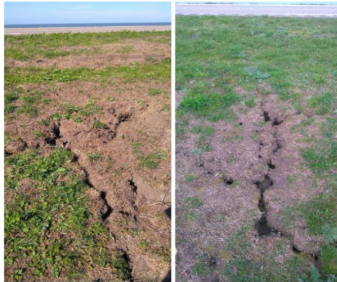
Figure 1. Cracks on 'Oostvaardersdijk'. Left: 1 month after drought. Right: 9 months after drought (Bottema et al., 2019)
