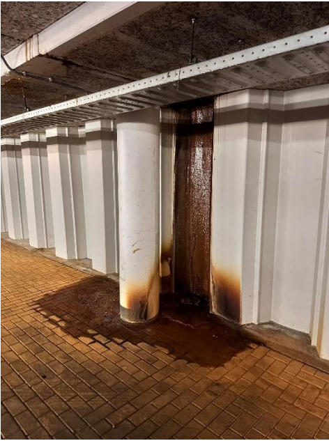
Figure 3.5. Water leakage P6.
