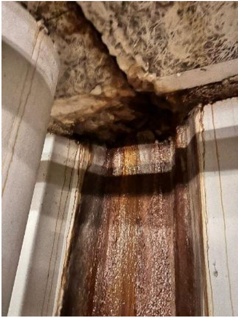
Figure 3.4. Water leakage P6, zoomed in.
