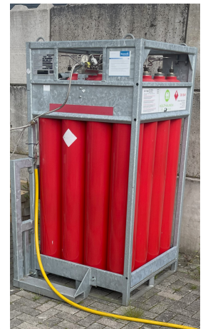
Figure 25: Gaseous hydrogen storage container
