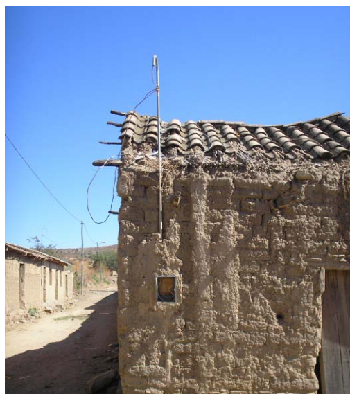
Non Payment consequences Electrification Phase II - Meter Removal -
