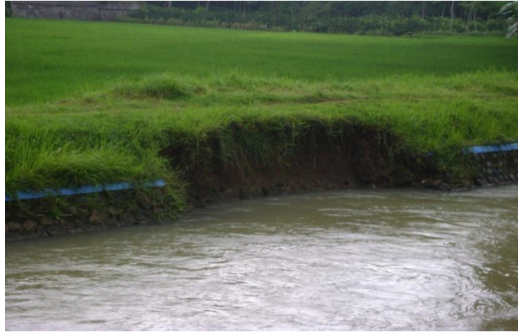
Figure 2.6b: Example of instability and erosion of outer slopes embankment primary irrigaton channel Boro
