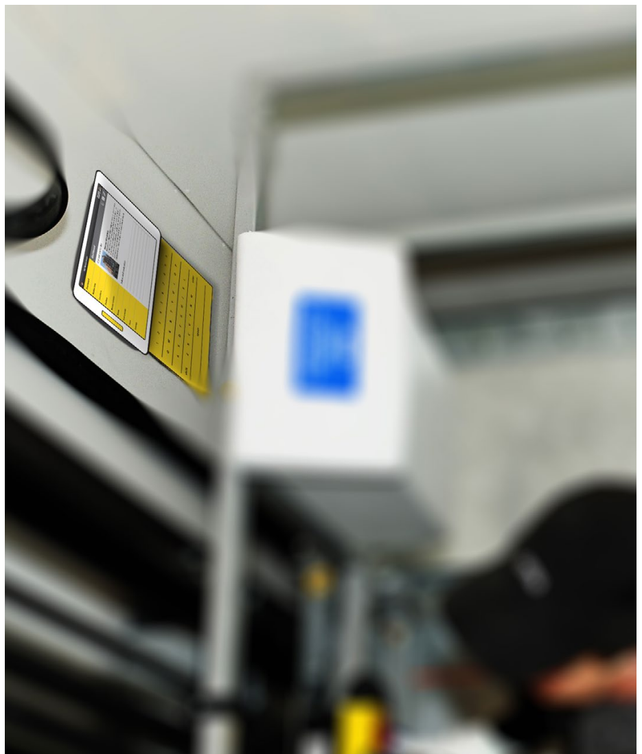
Figure 4.30: Tablet in elevator shaft
