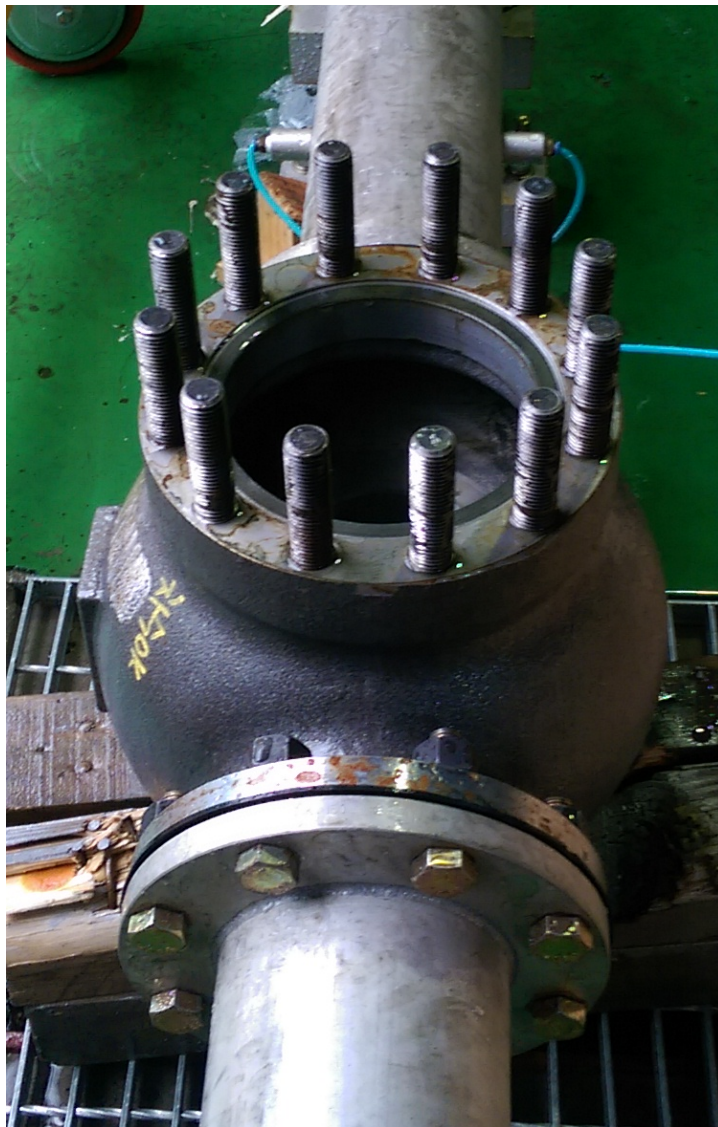
Figure 5.3: Empty valve body installed in the 6" - DN150 piping. Note the pressure tapping at the top of the picture for the upstream pressure gages.
