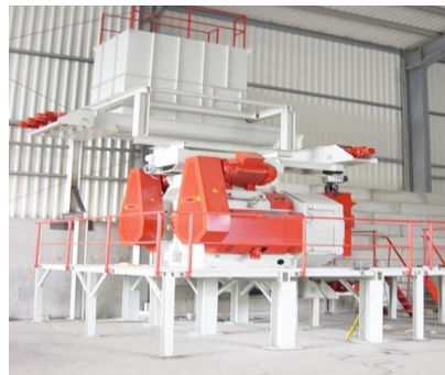
Figure 1.2: Installed production line in Germany
