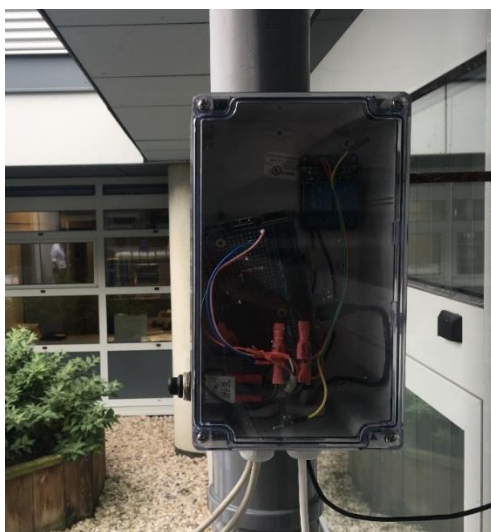
Figure 31: All electronics fitted in a single enclosure
