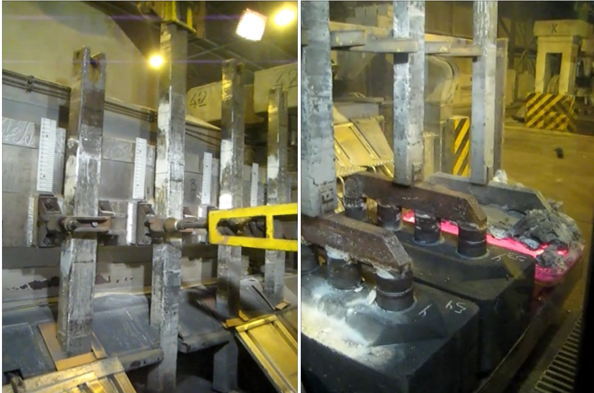
(A) Beam raising. The anode need to be repositioned on a daily basis in the electrolytic-cell. After the rod is disconnected, the fresh anodes and the one on the right is realigned in the cell. (B) Anodes including their rods. The two anodes on the left are basis in the electrolytic-cell. After the rod is disconnected, the fresh anodes and the one on the right is an used (still scorching) anode.
