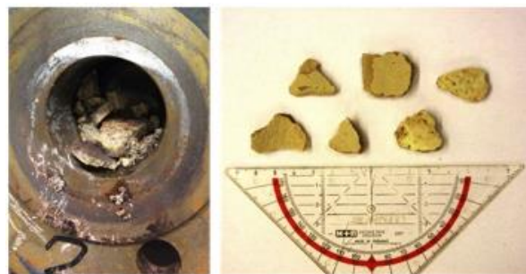
Figure 1.4 Deposits in piping of retort v14
