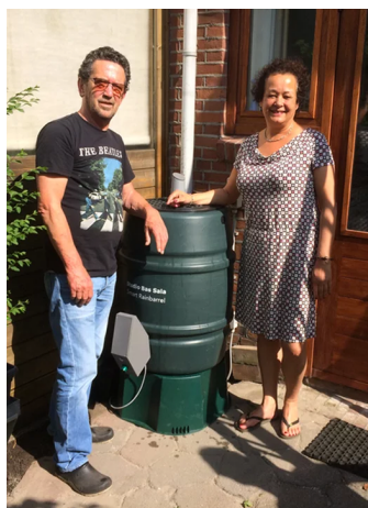
(b) One of 25 consumer oriented smart rainwater buffers installed by Bas Sala
