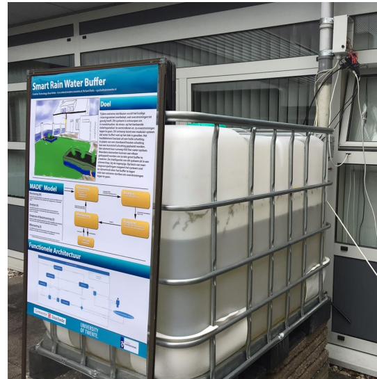
(b) The smart rainwater buffer prototype designed by Vetter
