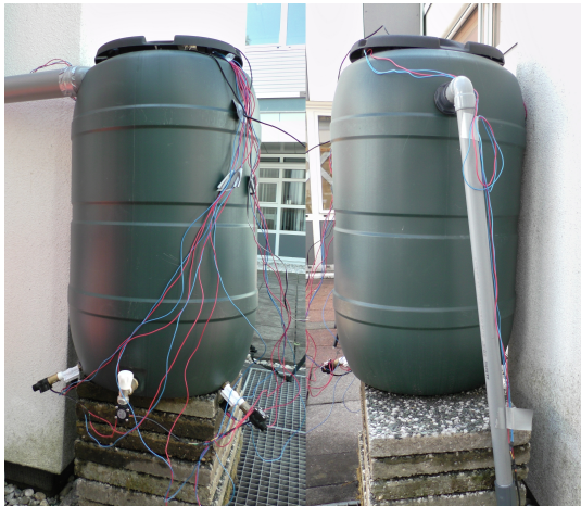
(a) The smart rainwater buffer prototype designed by Steeghs and Rindt
