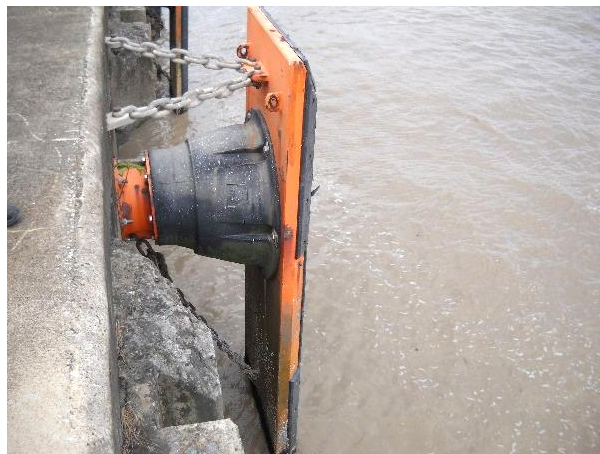
Figure 4.4 - Fender with damaged face pads, January 2018.
