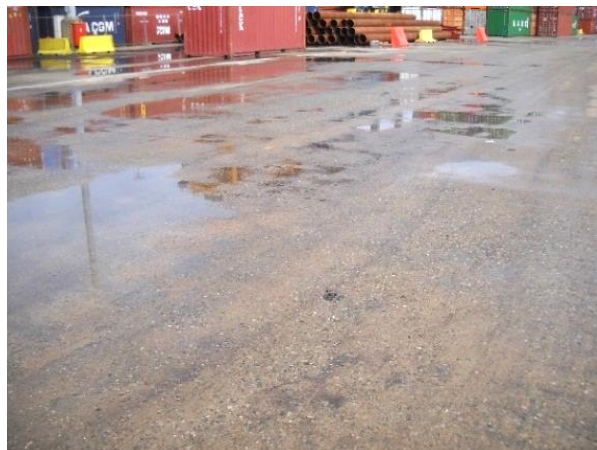
Figure 4.2 - Water puddles and sand on quay, January 2018.
