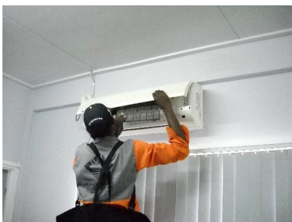
Figure 4.6 - AC unit filter cleaning, January 2018.
