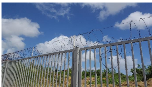
Figure 4.7 – Repainted fence and damaged razor wire, January 2018.
