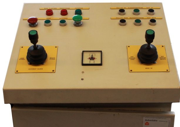
Fig.69: Jet-bridge operation panel
