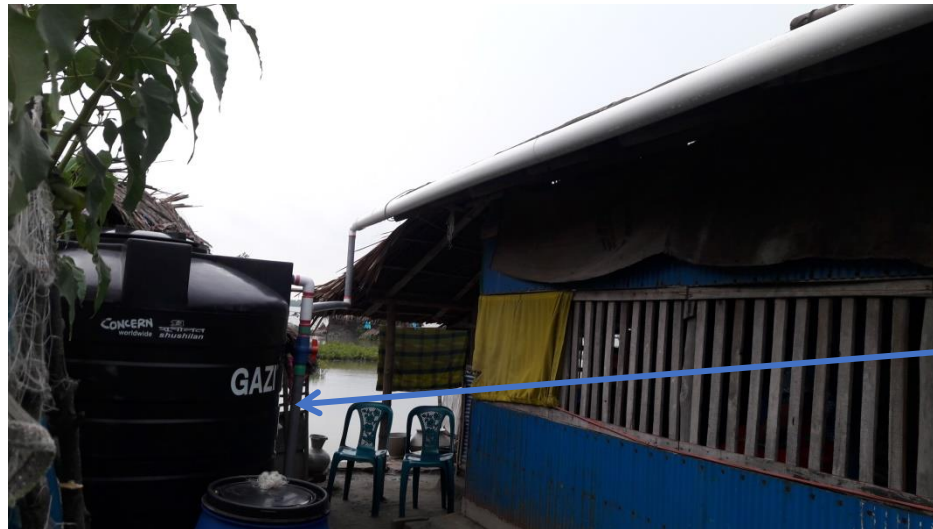
Figure 3.6: Foul water diversion pipe (Source: field data)
