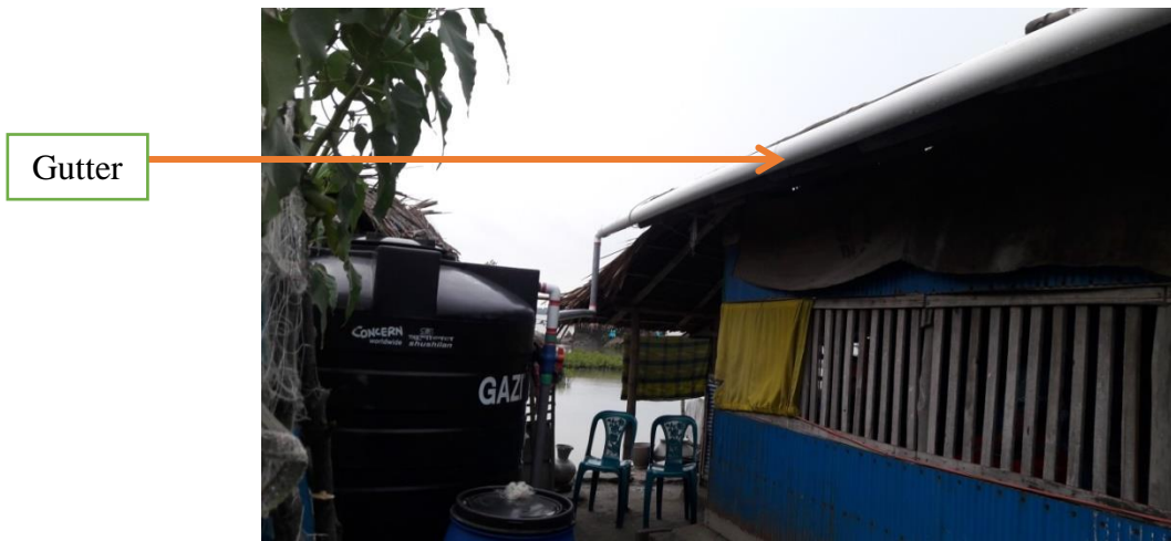
Figure 3.2: Guttering system of rainwater harvesting system (Source: field data)
