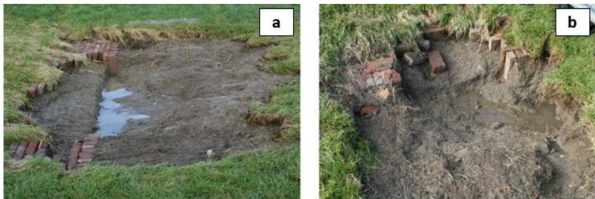
Figure 2.5 Grass cover erosion at the landward toe at test sections (a) Boonweg 1 and (b) Boonweg 2 after wave overtopping tests with a maximum mean overtopping discharge q_m = 75 l/s/m. Figures obtained from Van der Meer (2014).
