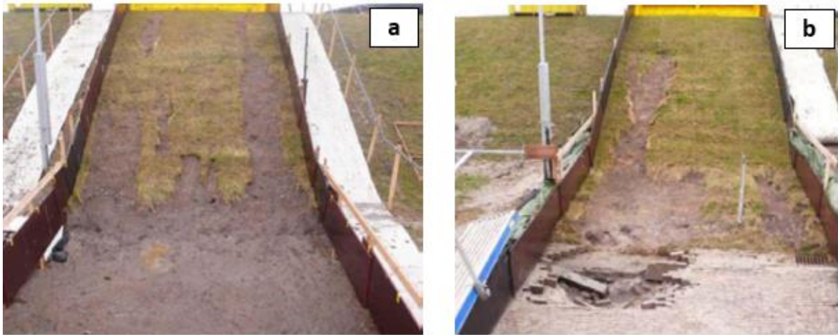
Figure 2.6 Grass cover erosion at the slope and the landward toe at test sections (a) Afsluitdijk 1 and (b) Afsluitdijk 2 after wave overtopping tests with maximum mean overtopping discharges q_m = 75 l/s/m and q_m = 10 l/s/m. Figures obtained from Van der Meer (2014).
