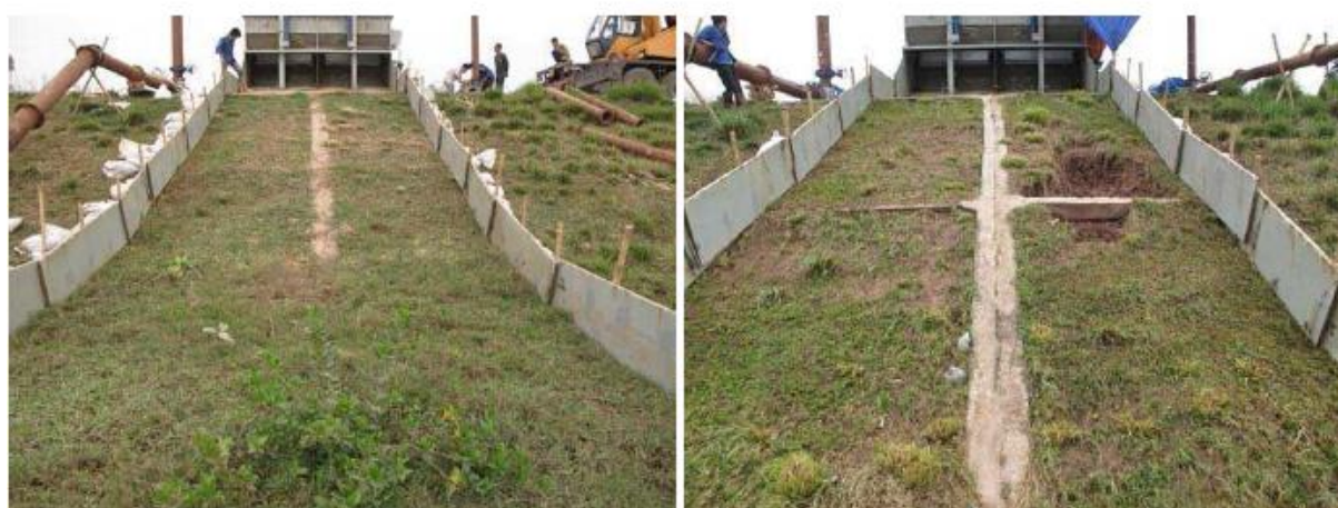
Figure A1.1 Presence of a concrete frame with horizontal and vertical beams in the grass revetment at Thai Tho, Vietnam, before testing (left) and after testing (right). Figure adapted from Le (2011).
