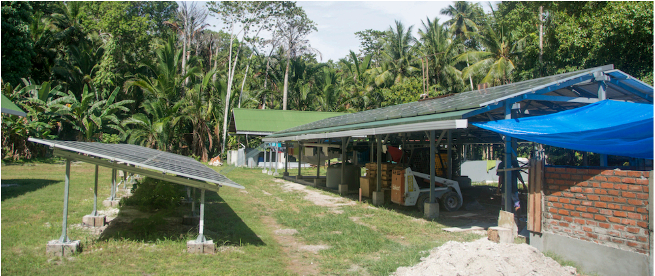
Figure 2: PV system at RARCC.
