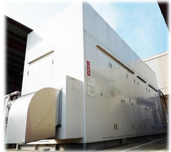
150°C heat supply HP (casing)
