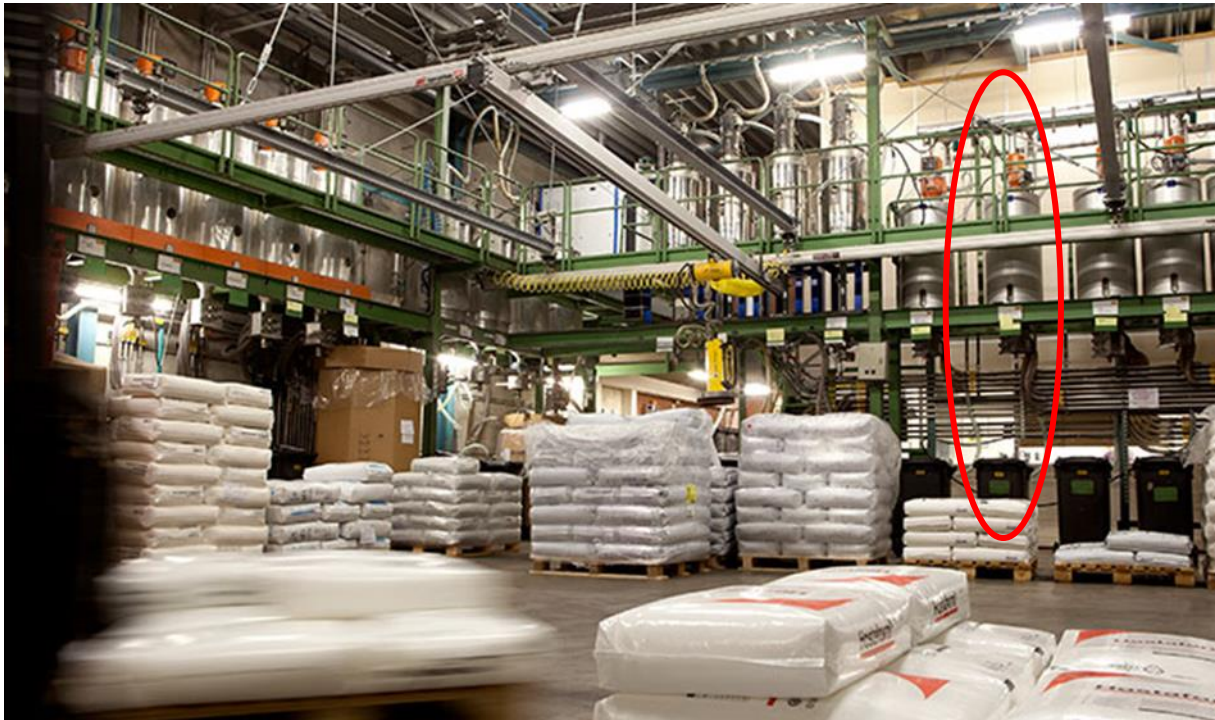
Figure 2.4. Raw materials warehouse with tube system
