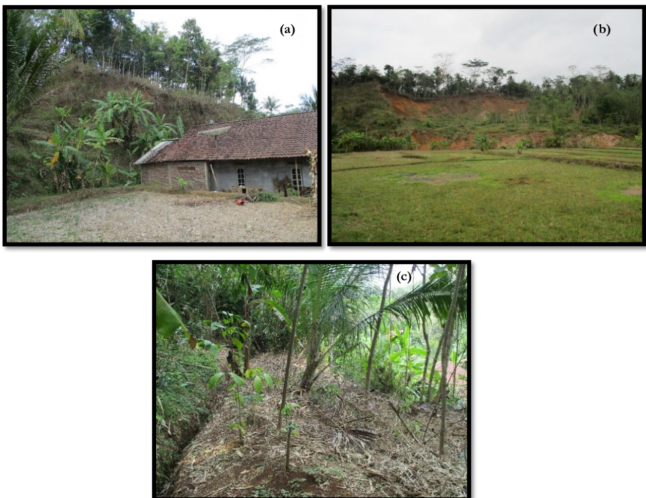
Figure 3-3 Landslides at Bompon and mitigation measure. One of the houses that were hit by the cut slope instability in 2011 (a), Deep-seated landslide (b), The drainage ditch along the slope (c)
