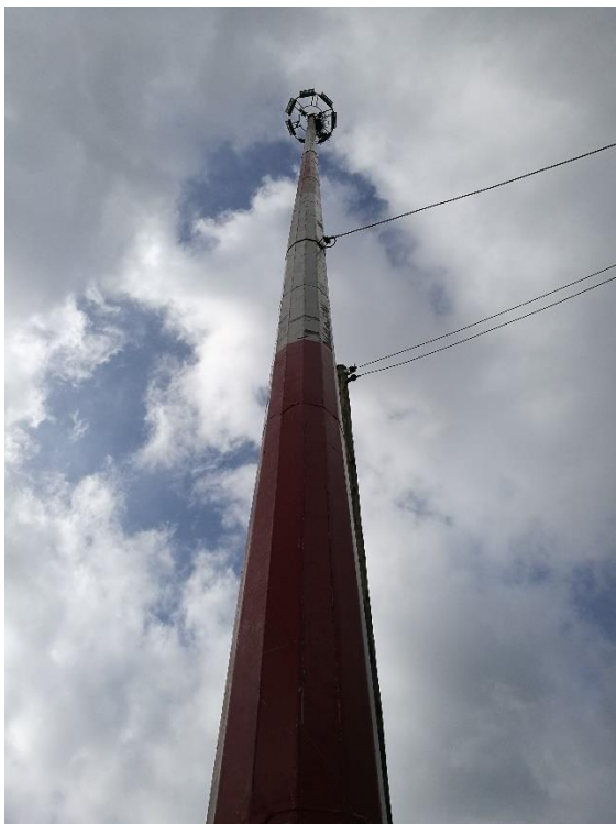
Photo 5a Big floodlight
