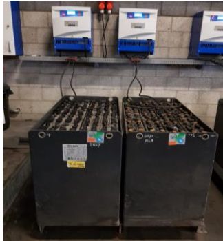
Figure 28 Two of the charging points and the equipment to charge the batteries.
