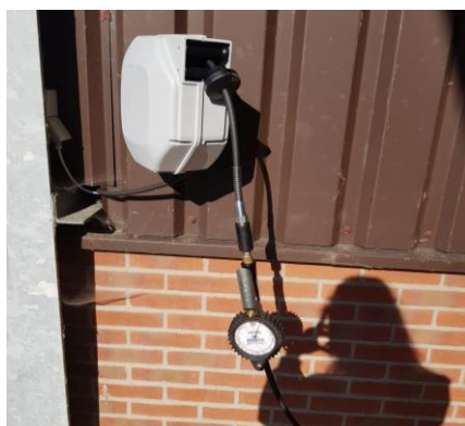
Figure 32 The part of the air compressor that is visible from the outside.
