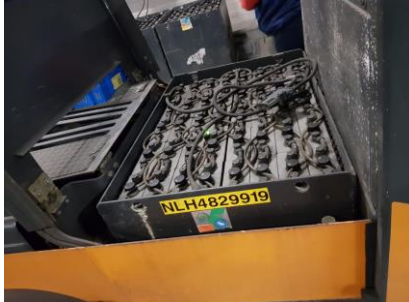
Figure 26 The battery in the electric car.
