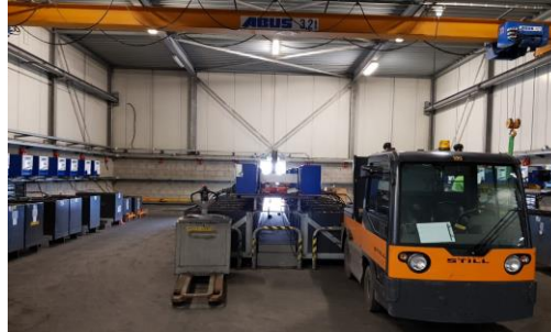
Figure 27 The charging station of all of batteries.
