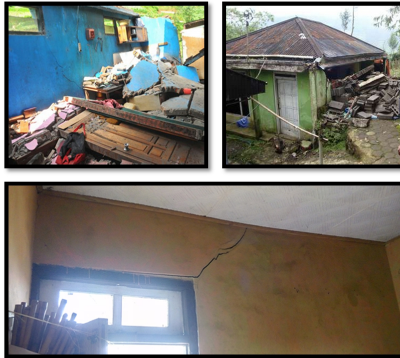
Figure 5.24. The impact of earthquake in April 2013, from small crack to collapsed house (antaranews.com, detik.com, and private documentation)
