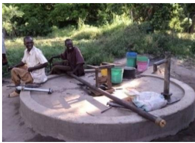
Functional need repair Nira/Tanira shallow well under rehabilitation at Kisaki ward Gomero village in Morogoro rural district.
