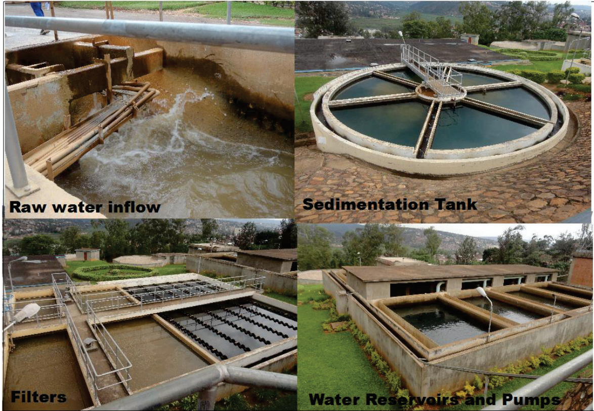
Figure 3-5: Infrastructure of Kimisagara water treatment plant
