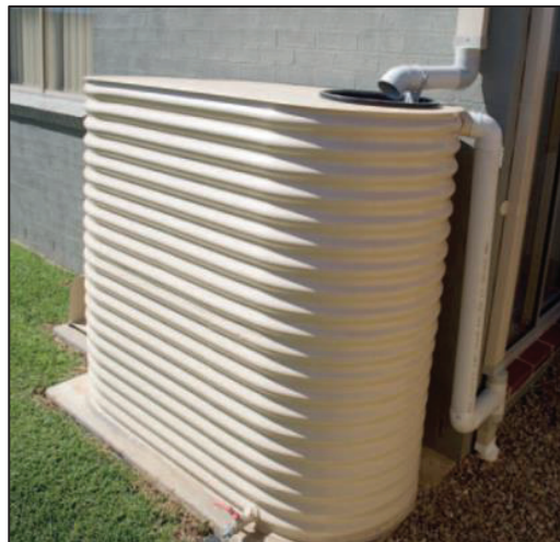
Figure 5-8. Rainwater harvesting tanks. Source (LANDCOM, 2009).
