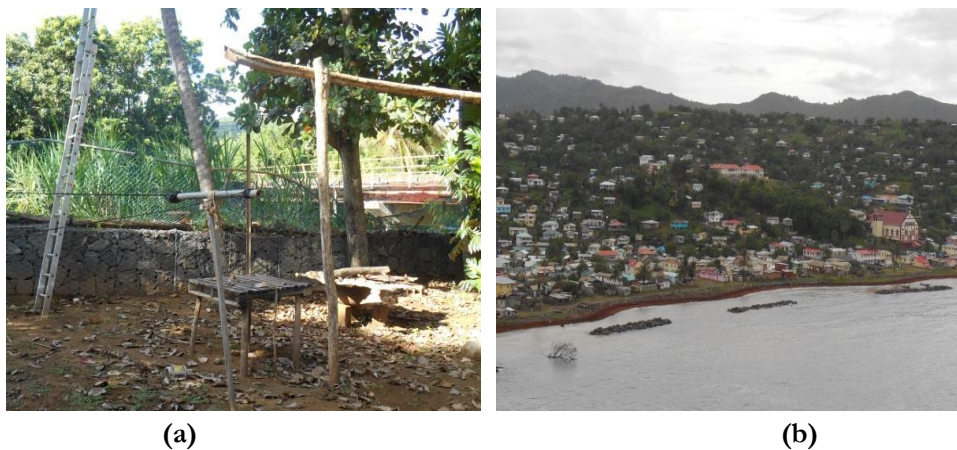
Figure 6-3: Structural mitigation work (a) Dennery (Mole) River dyke (b) Embankment at the sea
