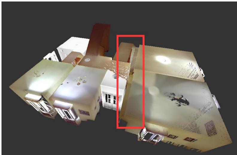
Figure 5-3 Some parts of the ceiling are not in the same plane with the others
