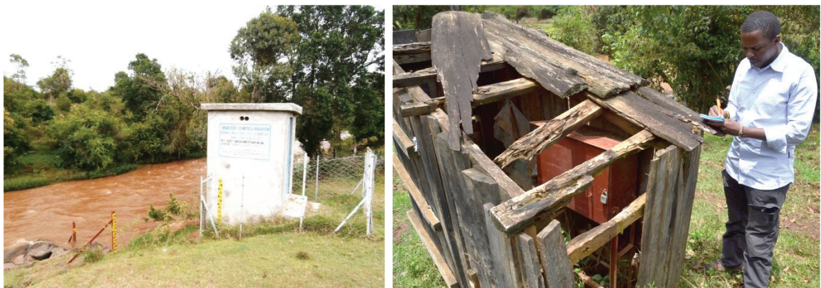
Figure 3: The picture on the left is Amala RGS at Kapkimolwa, Mulot. The station was rehabilitated and equipped with an automatic gauge with support from the World Bank Nile Basin Initiative (WB-NBTF), Swedish International Development Cooperation Agency (SIDA) and the Germany Society for International cooperation (GIZ). The picture on the right is neglected RGS at Emarti bridge along the Amala river. Picture by: Vekerdy Z.
