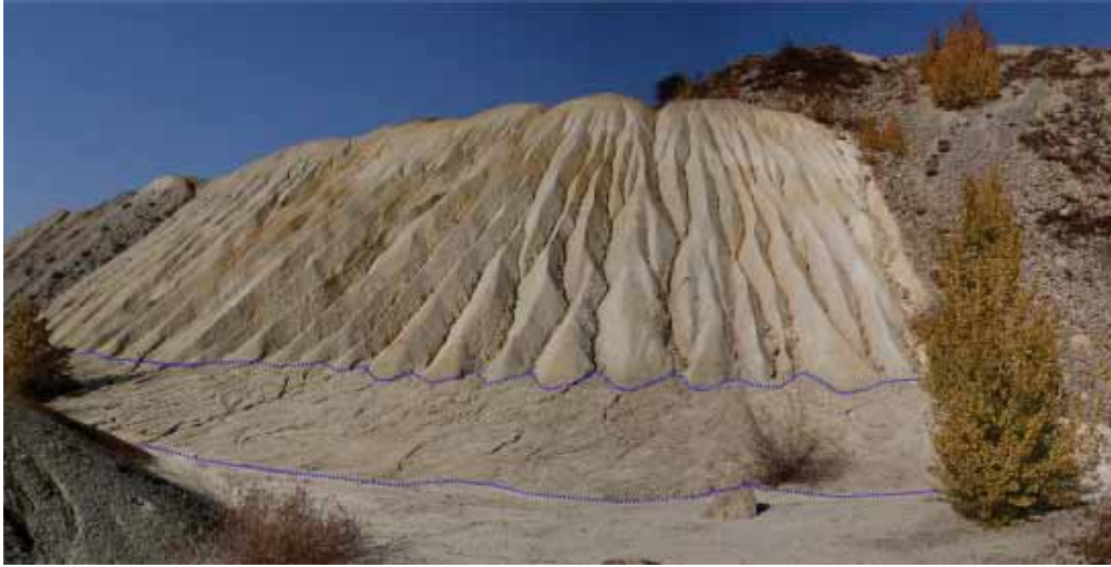
FIGURE 2.5: Gully erosion due to water running off the slope of the Saraka overburden waste rock dump (chapter 3). The talus deposits are situated in between the blue dotted lines. [4th November 2011, Bor, Serbia (44°6'44.3" N; 22°7'32" E)]
