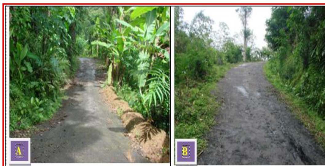
Figure 5.59: The alternative road condition based on community perception; A) The gebang to balai desa route B) The dangsembuh to gebang route (Source: Eko Setya N, 2011)
