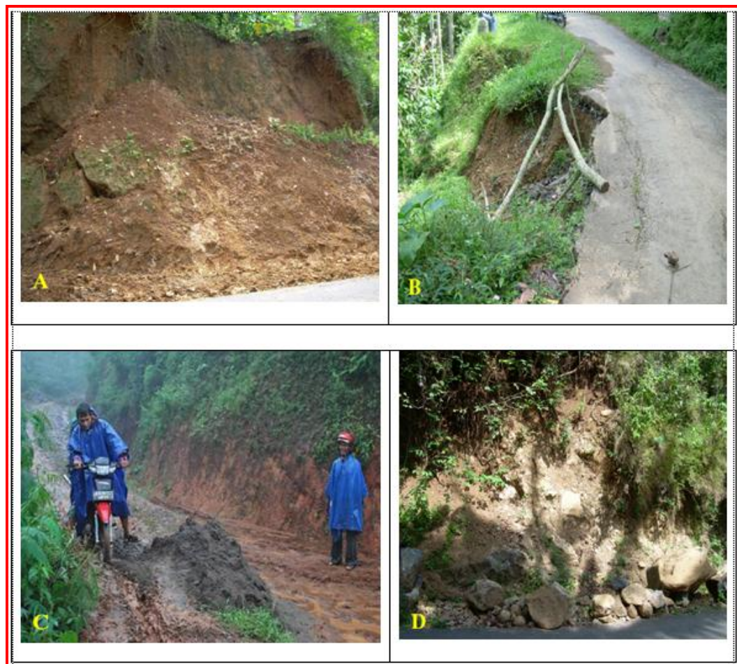
Figure 1.1: Road damaged due to landslide in Samigaluh District. A) Landslide covered Suroloyo road, Gerbosari in 2011, B) Suroloyo road, Gerbosari damaged due to landslide in 2011, C) Road damaged due to landslide in Balong, Banjarsari Samigaluh in 2010. (Source: KRjogja.com), D) Landslide type of rock fall that hit the regency road in Kebonharjo, Samigaluh in 2011. (A, B, D Source: Eko Setya N, 2011)
