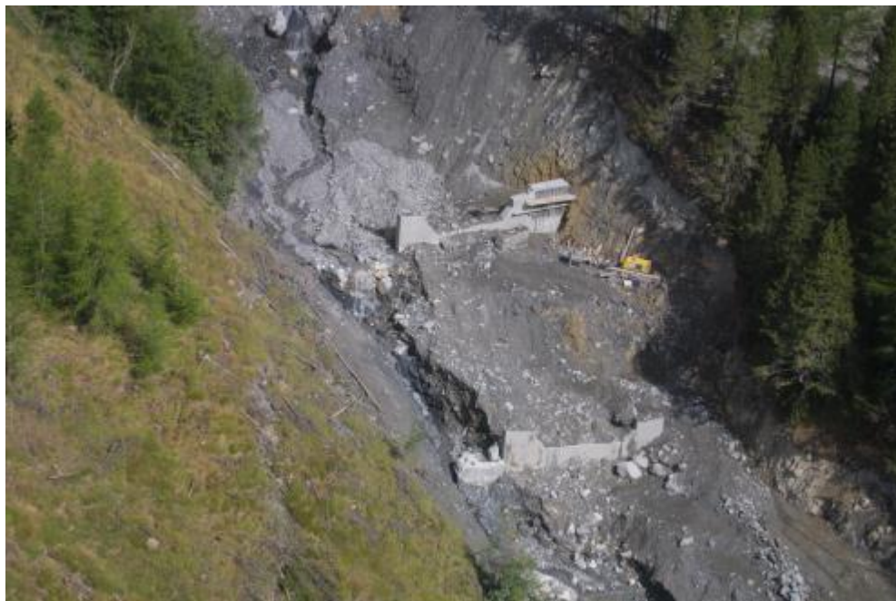
Damage to check dams at the entrainment zone
