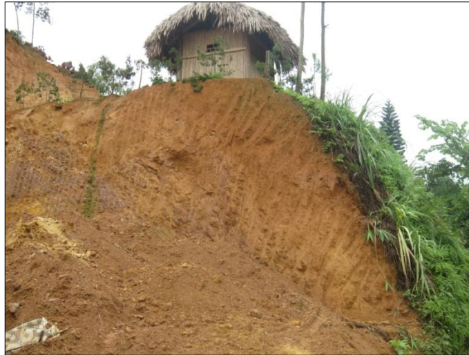
Figure 6-2: An example of putting load on the top of the slope (Khe Sen Street, Yen Bai)
