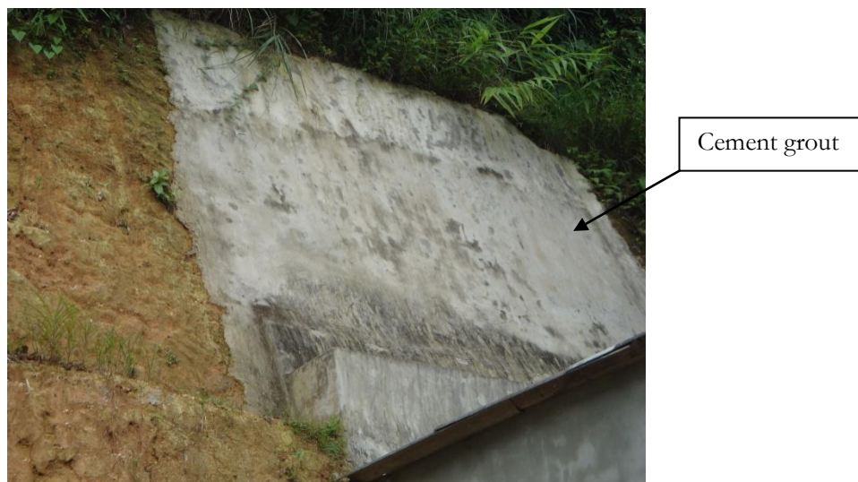
Figure 6-8: A simple type of slope surface protection in Cao Thang street, Yen Bai.
