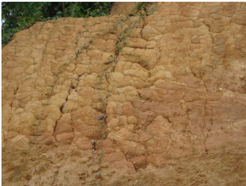
Figure 6-1: The development of cracks on a new cut-slope in group 45, Yen Ninh ward.
