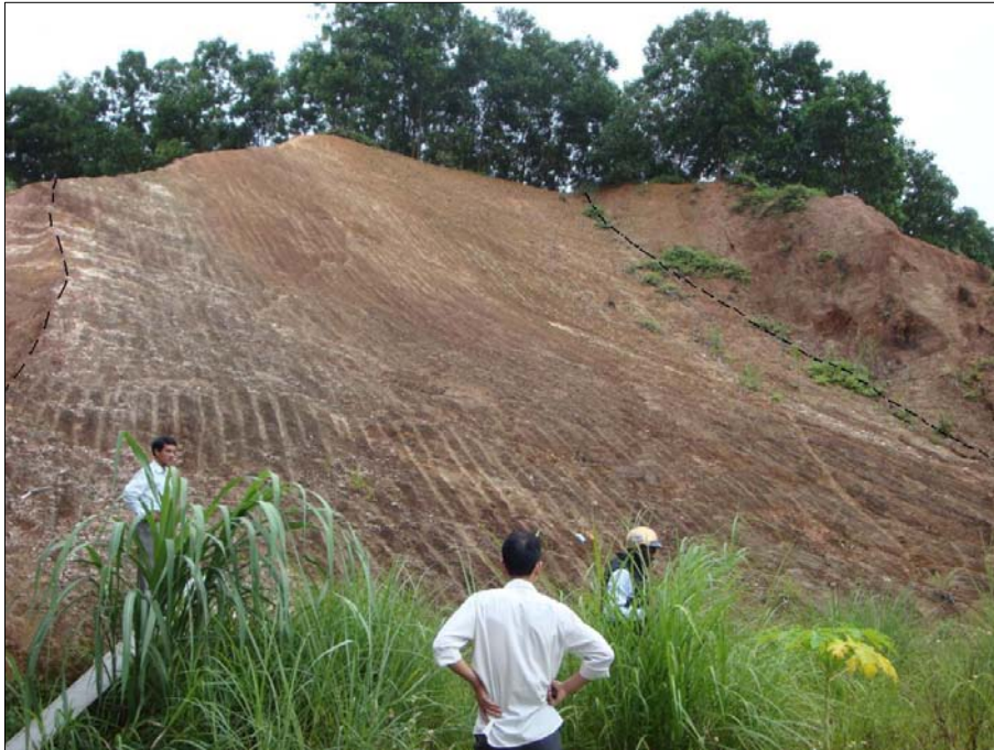
Figure 6-3: Cut to remove weathering production in Khe Sen street - Yen Bai
