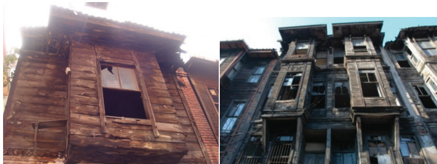
Figure 29 Listed timber buildings in a ruined and abandoned condition
