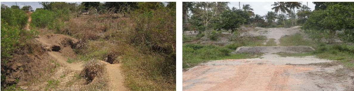
a) Poorly constructed road with no culvert-Mivumoni b) Poorly finished road with a small culvert-Buyuni
