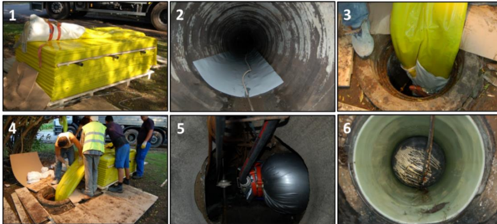
Figure 3: The process of CIPP lining to renovate a sewer section. Source: (Almeida, Covas, & Beceiro, 2015)
