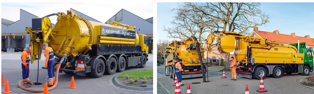
Figure 5: Sewer cleaning using a combi truck (left) and two separate vehicles (right). Source: (vandervalk+degroot, n.d.)
